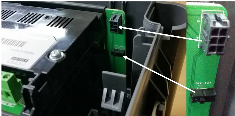
Figure 12. Battery On/Off Switch and Battery Connector
